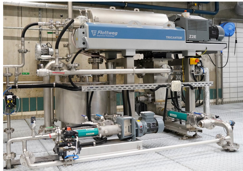
The Tricanter® is the heart of systems used to process cooking oil, separating the old cooking fat into water, oil, and solid particles.
